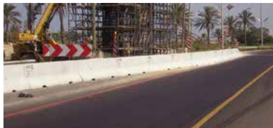
Haifa southern approach. Temporary mobile restraint system for the purpose of bridge construction work. Model: DB80/4M k180
